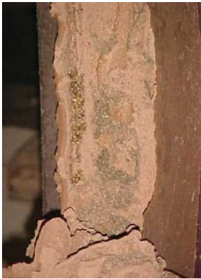
Picture: Dead termites above toilet
